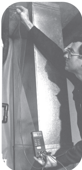
FIGURE 60 TEMPERATURE RISE MEASUREMENT
